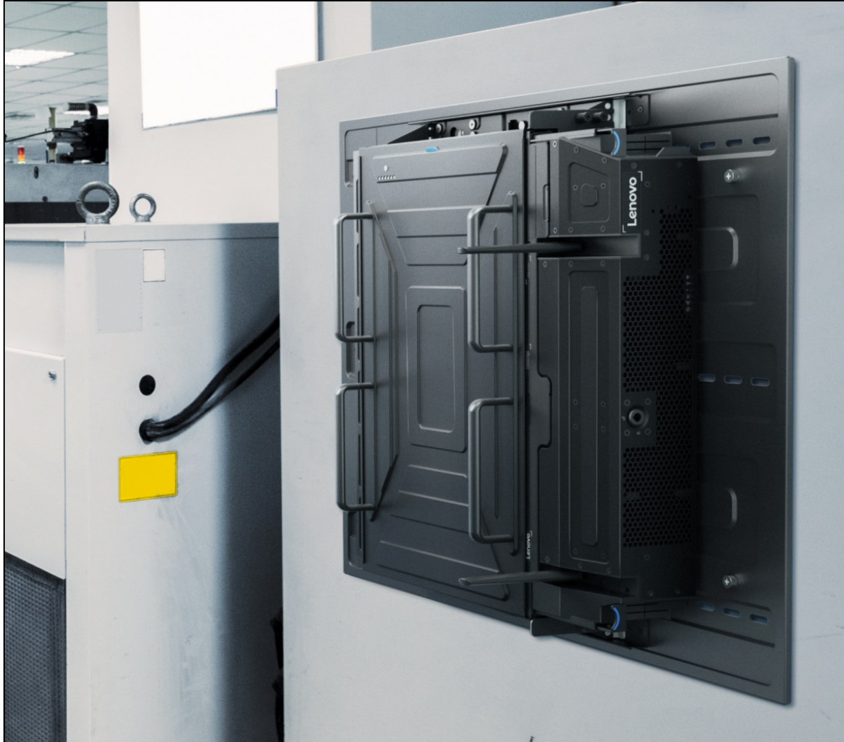
Figure 18. SE450 installed on a wall in a manufacturing environment
