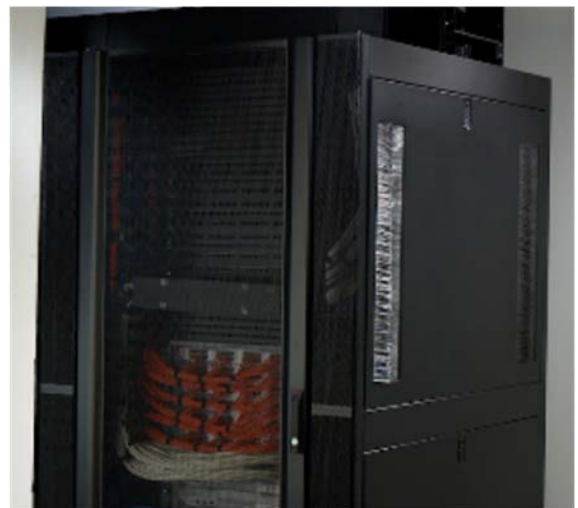
Installed on AR3340 enclosure
